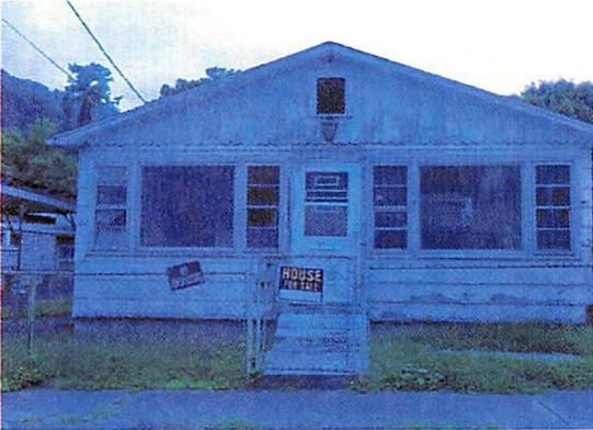
Parcel 2: Howard Avenue, Privately Owned, Vacant and Dilapidated
