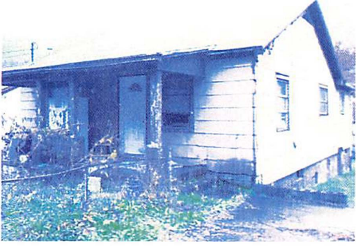
Parcel 22: Billy Hobbs Avenue, Privately Owned, Vacant and Dilapidated
