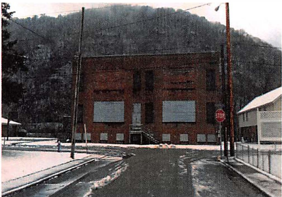
Oakland School and Gym, Kanawha Avenue, City Owned, Vacant and Dilapidated. Frontage on Kanawha River and available for development to support tourism.
