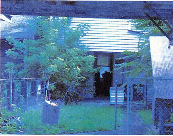
Parcel 170: Howard Avenue, Privately Owned, Vacant and Dilapidated
