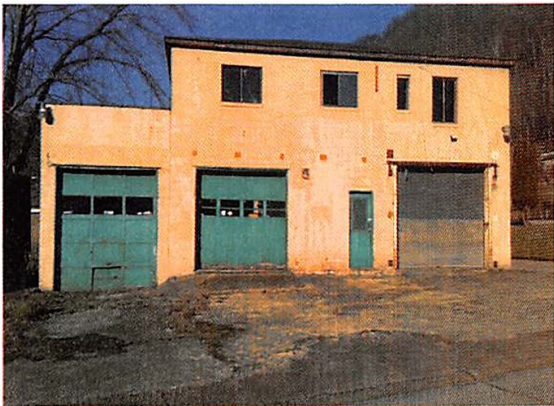
Michigan Avenue, Commercial, Privately Owned, Vacant and Dilapidated
