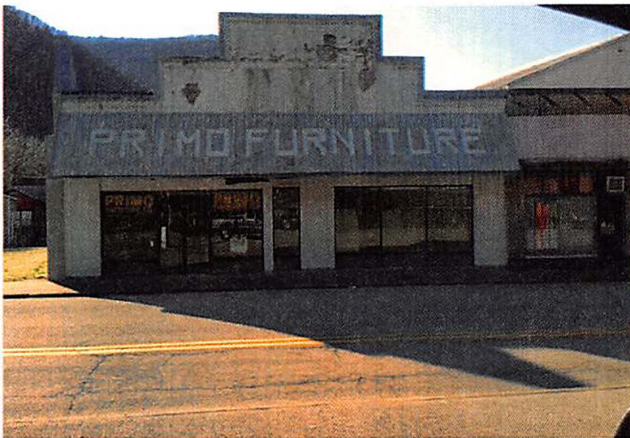
Michigan Avenue, Privately Owned, Commercial, Vacant, Dilapidated, recently broken into and windows are now boarded. Within view of Rt. 60.
