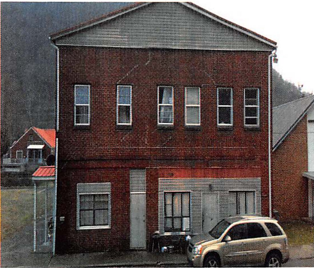
Michigan Avenue, Commercial, Privately Owned, Dilapidated, Chronic Ordinance Violations. Within view of Rt. 60.
